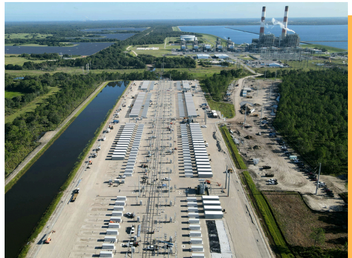
Manatee Solar's Battery Storage Site
